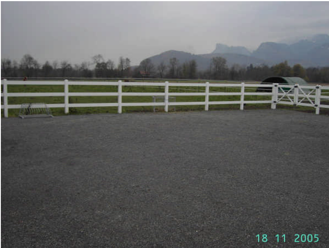
Photo 4: Horseback riding Dünser "grass concrete Ecoraster" Clear tread eastern area (east of the pit / of forecourt according photo 3), peripheral drainage drainage if necessary; 18.11.05
