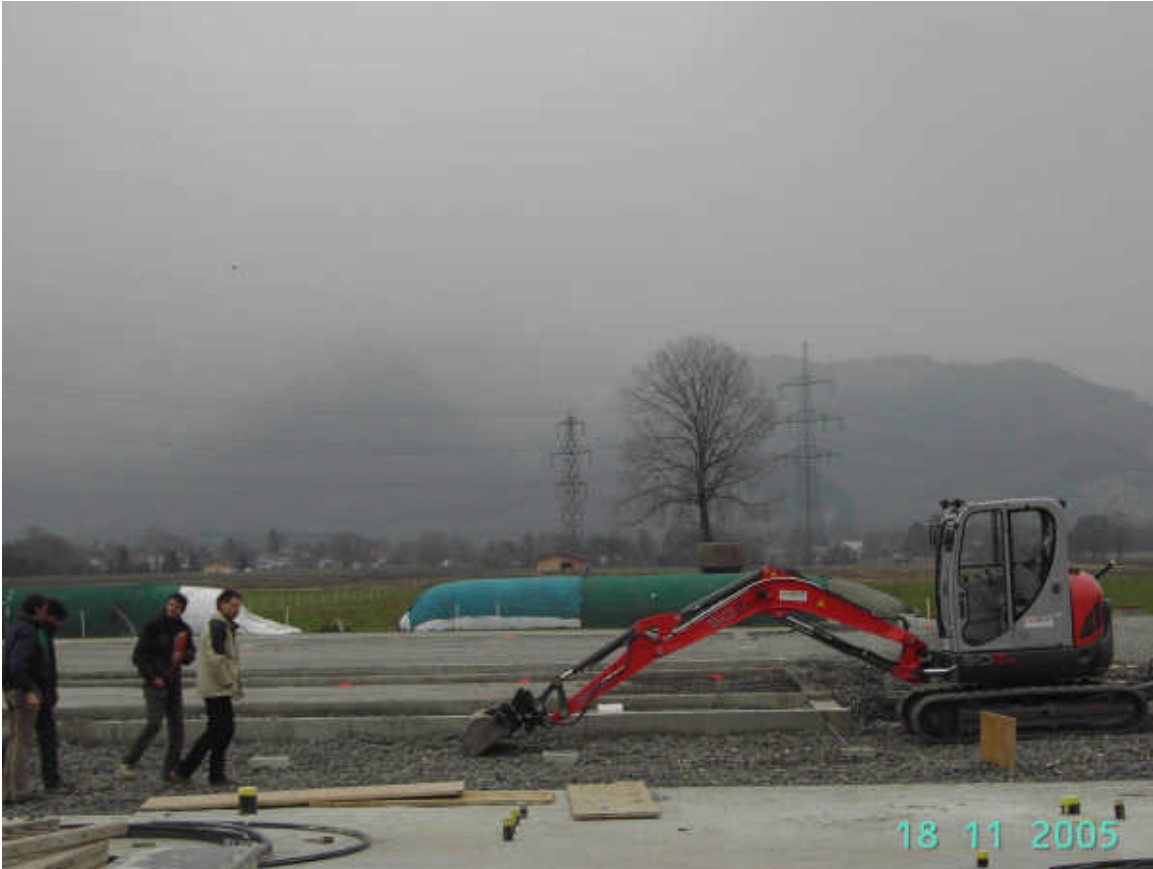
Photo 2: Detail Recording Reithof Dünser, looking towards the west, as of 18.11.05; Ummauerte areas behind excavator bucket seats are future boxing / Pedoks.
